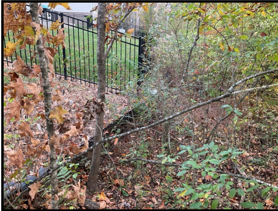
Photo 7 - View of the Unusual Condition and Comment (Object ID 12)
