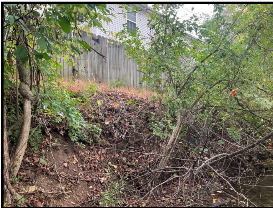
Photo 13 - View of Erosion Site
