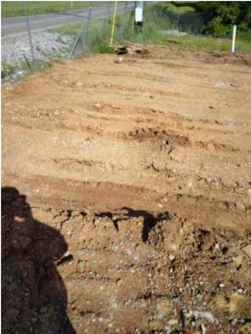
Proofroll material responded with rutting
